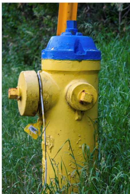
Figure 27. Fire hydrant painted according to the NFPA 291 colour code.
