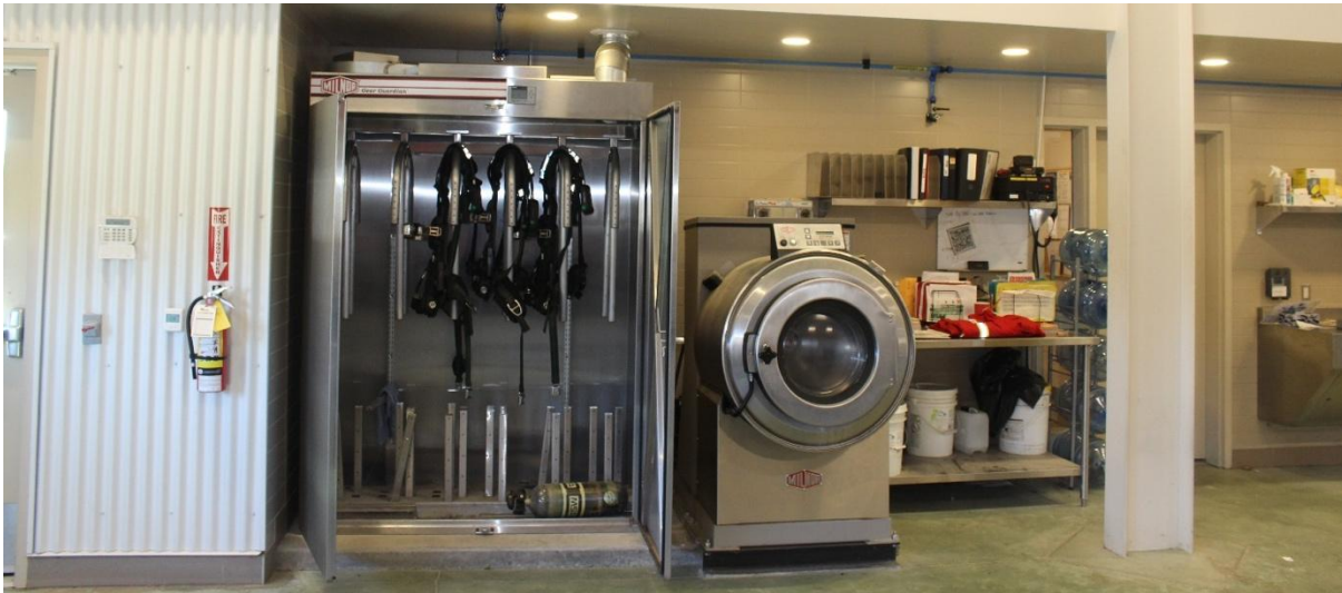
Figure 21. PPE extractor and dryer at Station 6 – Perth Road.
