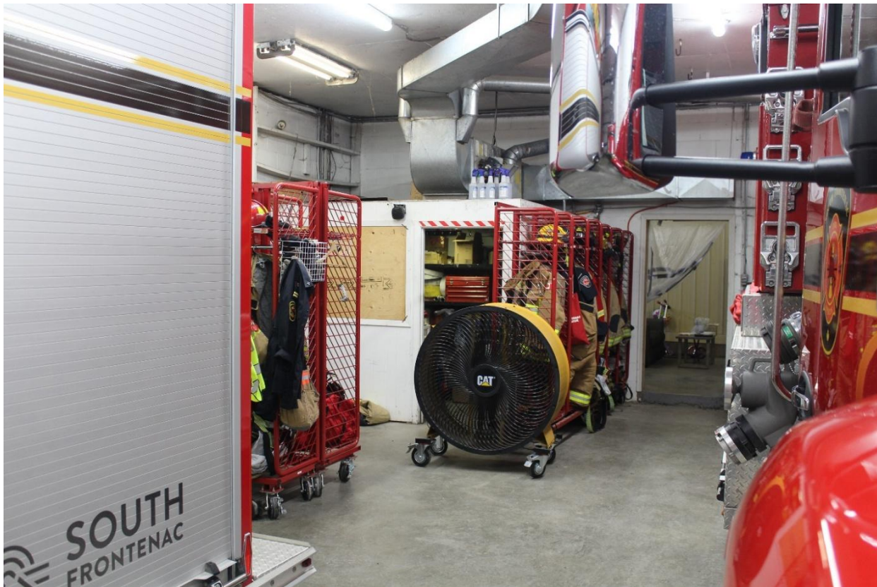
Figure 23. Fire apparatus area at Station 7 – Inverary.
